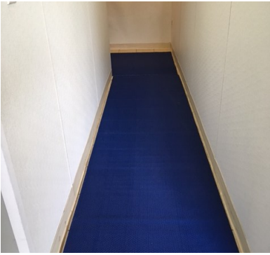
The restrooms are much safer now with new floor mats!
